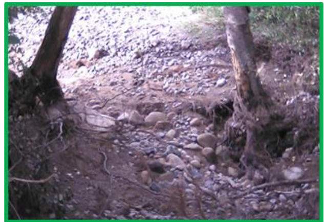
Close up of the exposed tree roots
